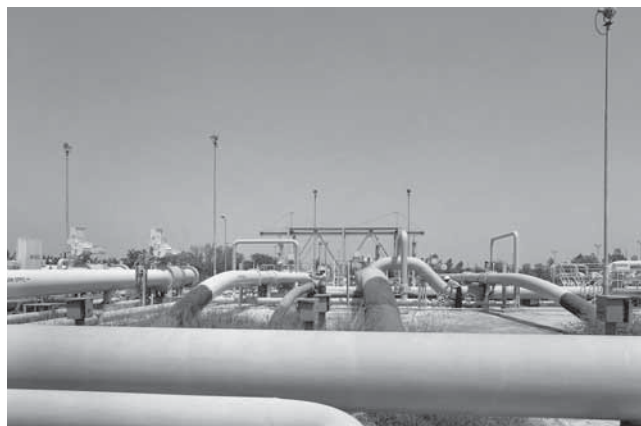
GAIL gas pipeline system
