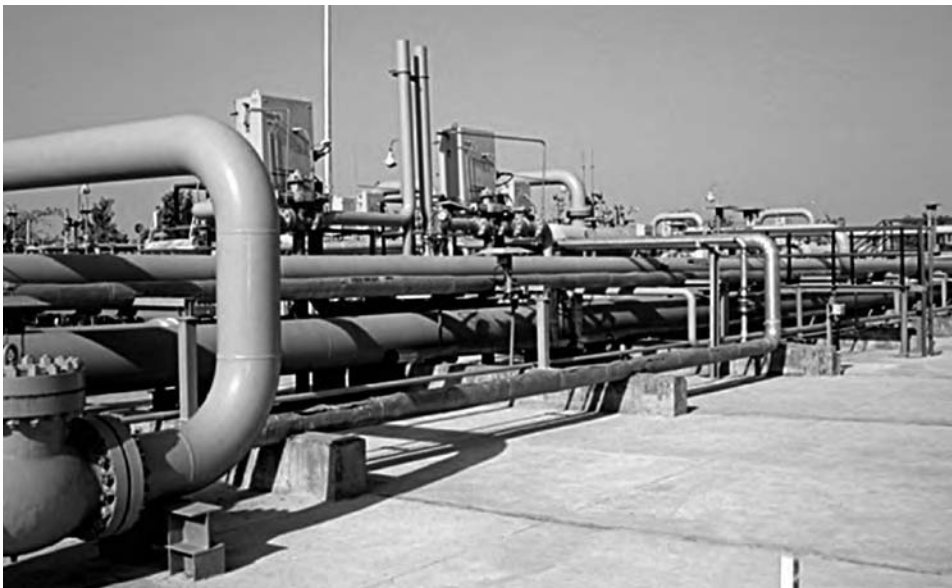
Gas Terminal Station
