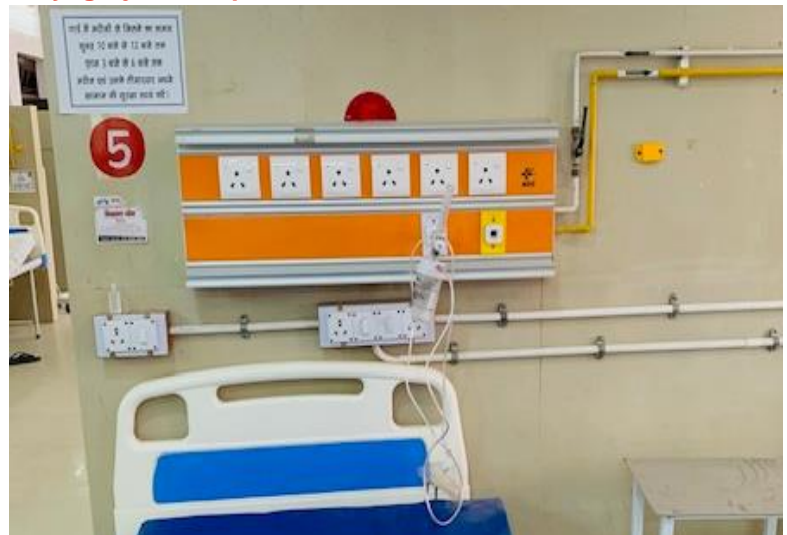
Figure 8: Head panels connected directly with PSA Plant in Prayagraj TB Hospital
