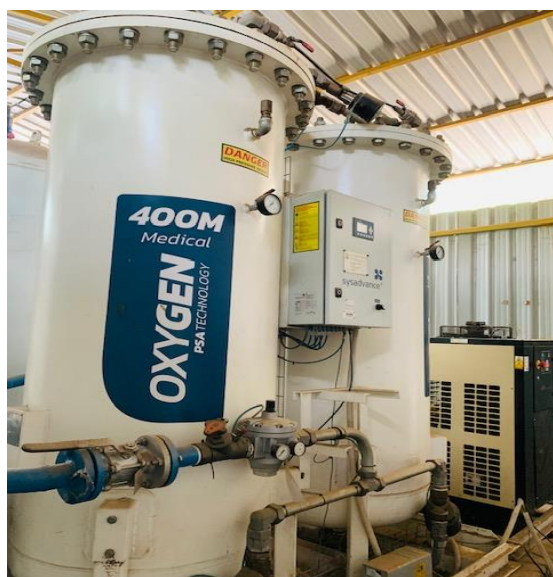
Figure 10: PSA Oxygen Plant of Guna district hospital
