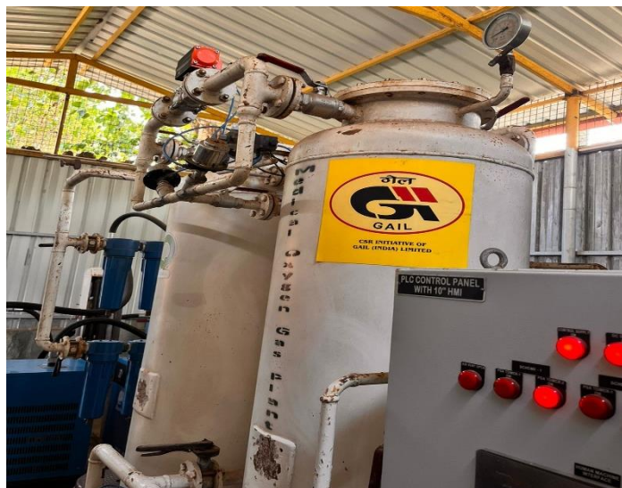
Figure 9: PSA Oxygen plant in Udupi district
