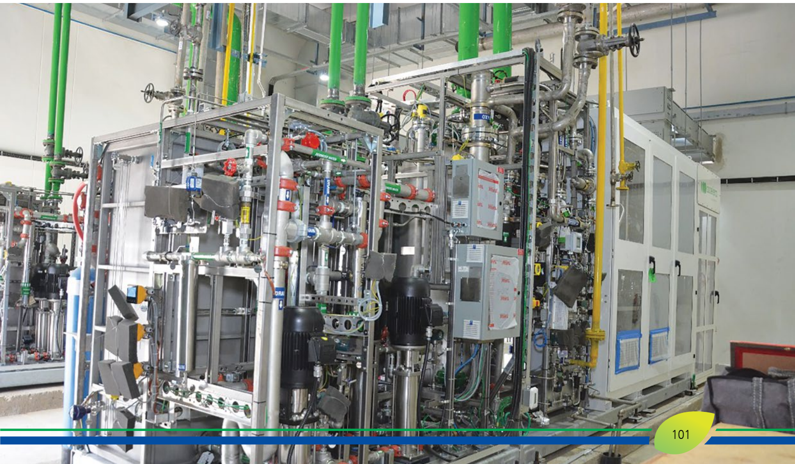
10 MW Green Hydrogen Plant in GAIL, Vijaipur
