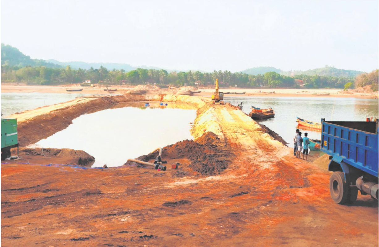
A cofferdam is being built across the Netravati in Mangaluru to facilitate laying of pipeline below the riverbed for the 438 km Kochi-Koottanad-Mangaluru Regasified Liquefied Natural Gas pipeline. The work is being executed by GAIL. ■ANIL KUMAR SASTRY
