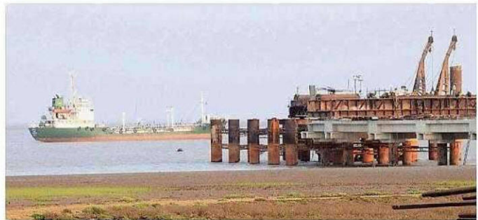
Dhamra LNG Terminal Pvt Ltd, a unit of Adani Ports and Special Economic Zone Ltd, is constructing a 12-million-tonne-per-annum LNG re-gasification terminal at its port
